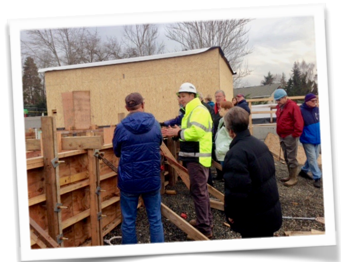
Mack Thames, Project Manager for TEAM, providing a tour of the construction site in December.
